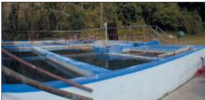
Photo 52. Cordillera potable water treatment plant in Ciales, Puerto Rico. Photo by L. Miranda Castro.
