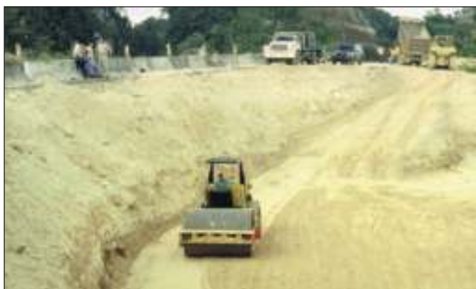
Photo 61. Maintenance activities in Highway PR 10. The road had already been officially opened when this picture was taken. Continuous landslides make it unlikely that this level of maintenance will ever abate in this road segment. Photo by L. Miranda Castro.
